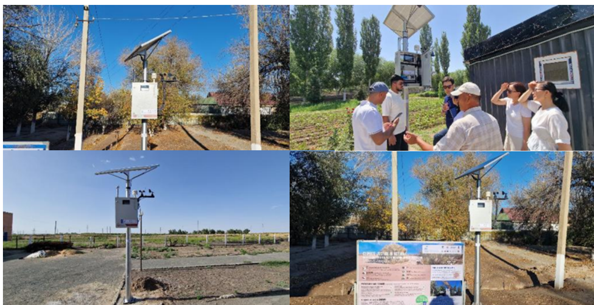
Photos 60,61,62,63: Established AQMS equipment in Karakalpakstan
